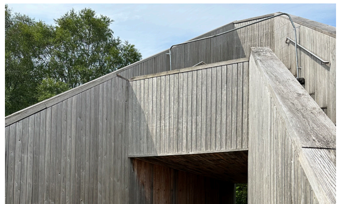
The Pyramid Viewpoint by BTE Architecture, current condition. (Photo credit: Jordan Silver)
